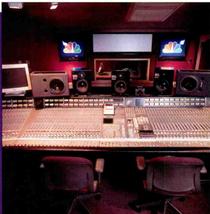
Edit 7 at NBC's New York facility serves as the music mix and post-production room for "Saturday Night Live," a program produced in matrixed surround sound.
